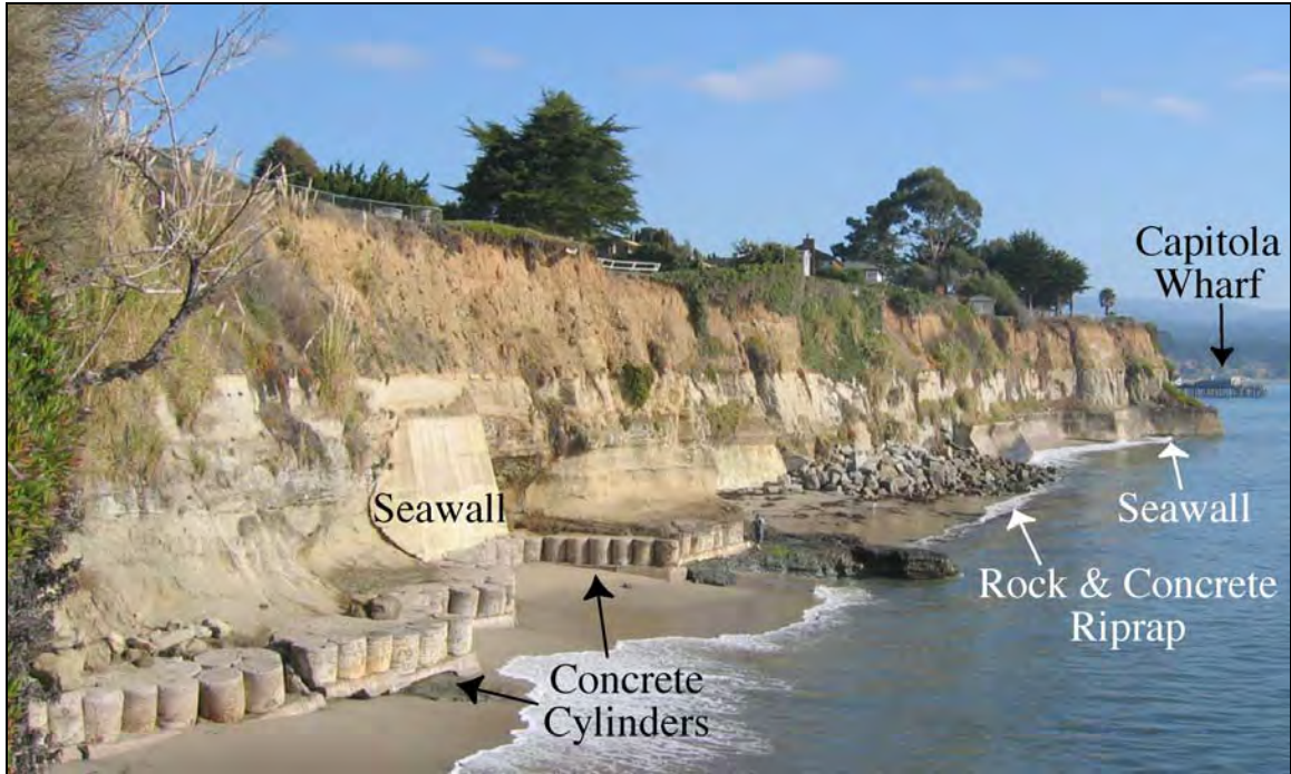
Figure 3: An unplanned assemblage of coastal armoring at Opal Cliffs in Capitola, California can have a visual impact on the beach user.
