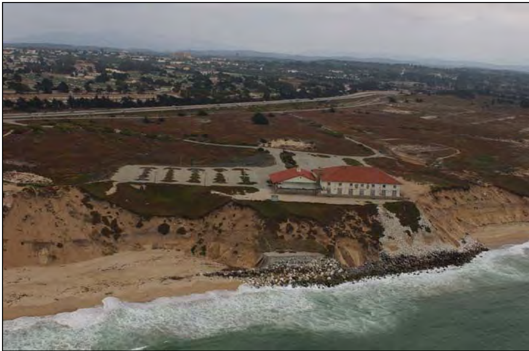
Figure 1a: Oblique aerial photograph of Stillwell Hall in 2002 in Marina, CA. Coastal protection structures placed at the base of the aged building were neither effective nor efficient enough keep up with intense coastal erosion of adjacent bluffs. Photograph copyright © 2002 Kenneth & Gabrielle Adelman ( http://www.californiacoastline.org/ ).
