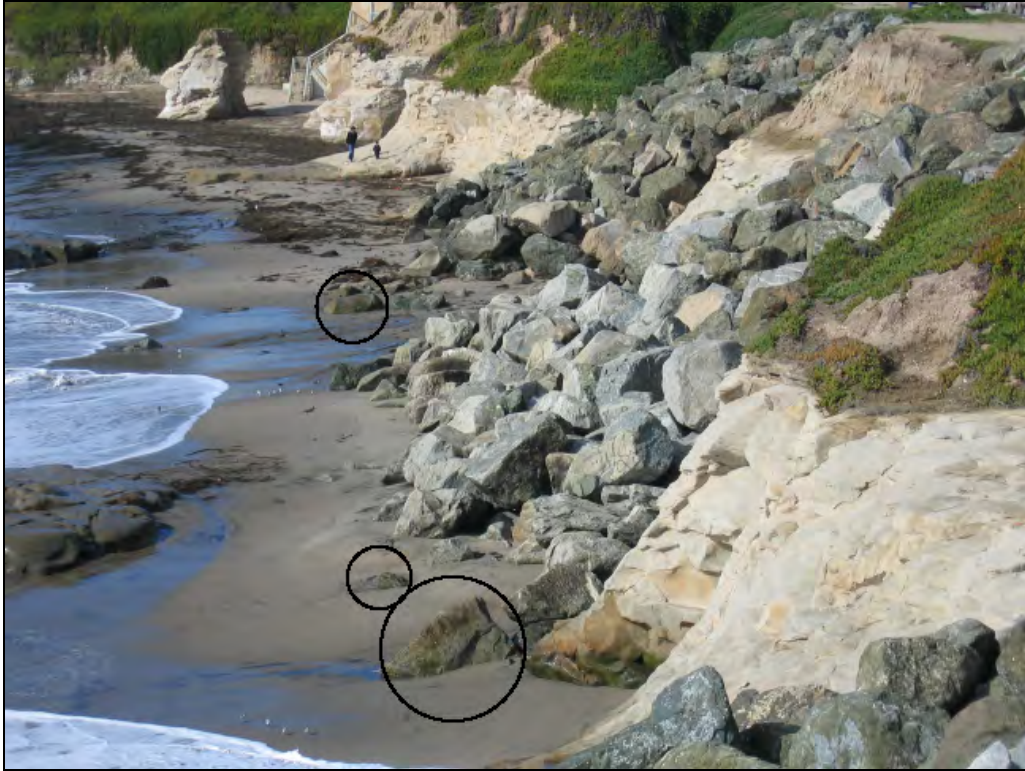
Figure 9: Riprap boulders commonly settle into deep sandy beaches or get buried, as seen here near the intersection of Westcliff Drive and David Street in Santa Cruz, California.
