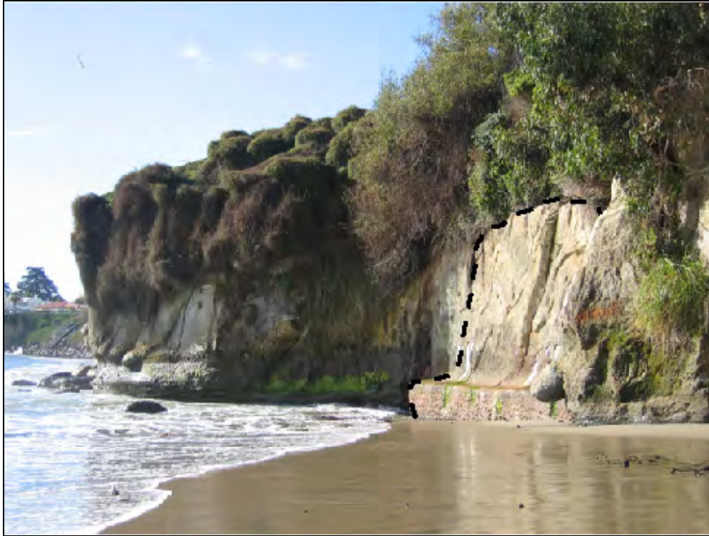
Figure 4: Photograph of cliff stabilization built to fill a seacave at Cowell's Beach in Santa Cruz. The 2004 gunite wall, outlined by the black dashed line, mimics the shape and color of the natural cliff.
