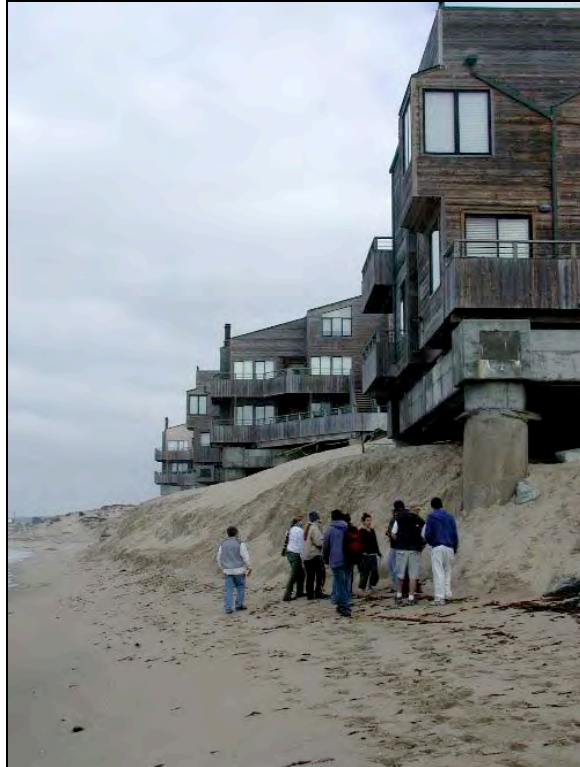
Figure 5.7: Exposed pilings at the Ocean Harbor House condominiums in Monterey. Photo: Doug Smith, CSUMB.
