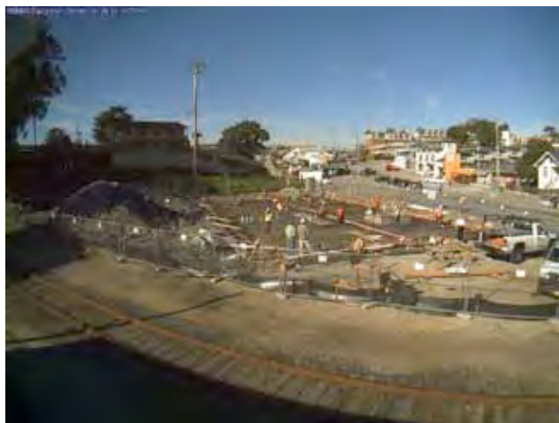
Image of the Sanctuary Exploration Center Construction site from the live webcam.
