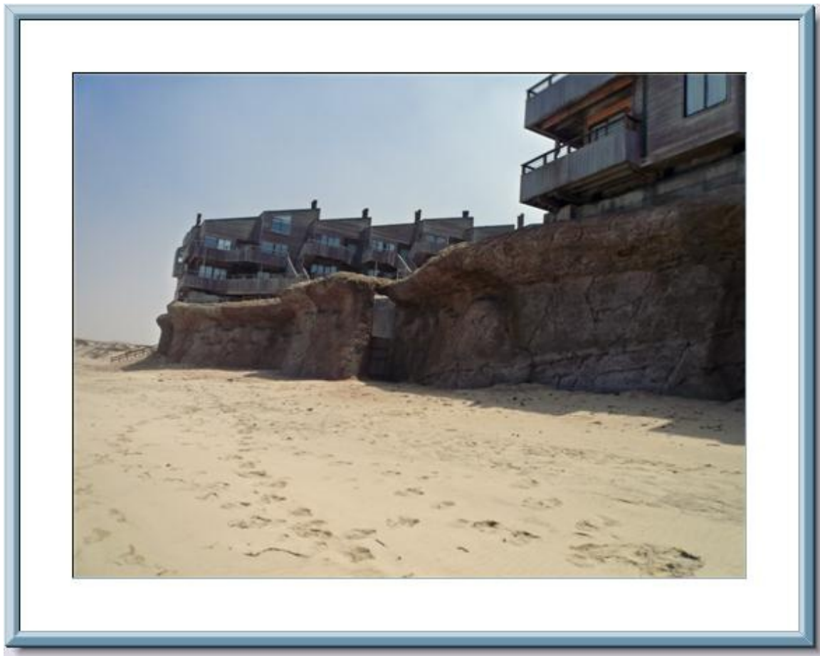
Figure 41 Example of a seawall, Ocean Harbor House, Monterey, CA (Photo Gary Griggs)
