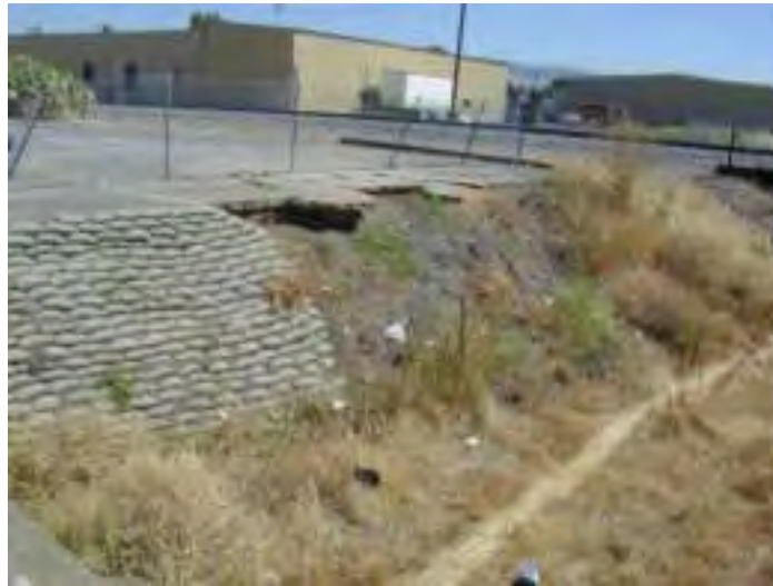
Figure 4.35. Bank and parking lot erosion east of Monterey Road on Upper Miller Slough.
