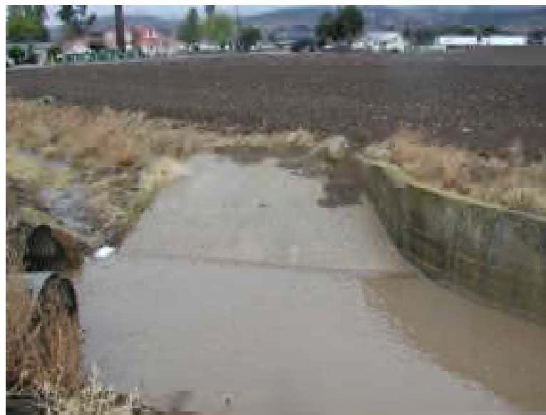
Figure 5.4. Example of Channel Modification and Vegetation Removal related to Agricultural Hydromodification.
