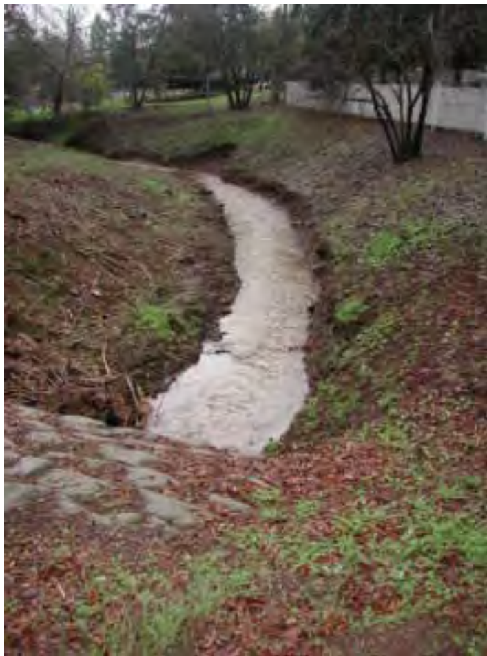
Figure 4.20. Bank failure on Paradise Creek on Llagas Road.
