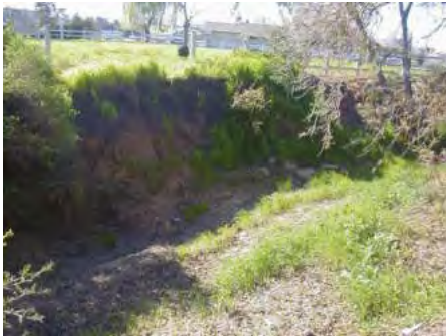
Figure 4.23. Bank erosion downstream of Columbet Avenue where water re-enters the channel from upstream into San Martin Creek.
