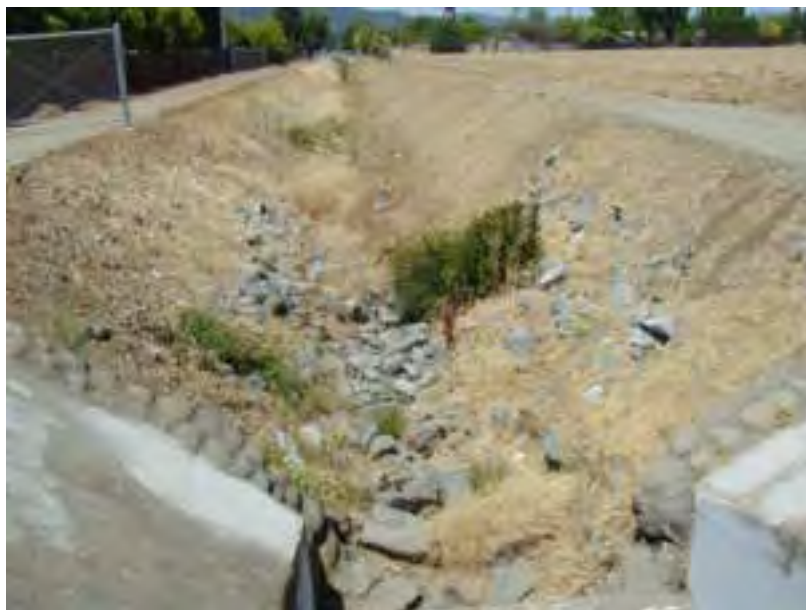
Figure 4.48. Riprap slumping into Princevalle Drain upstream of Monterey Highway.
