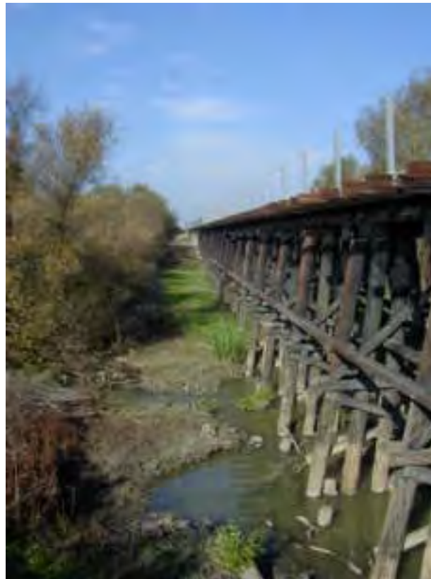
Figure 4.45. The Pajaro River at the Southern Pacific Railroad trestle, south of the confluence with Llagas Creek.
