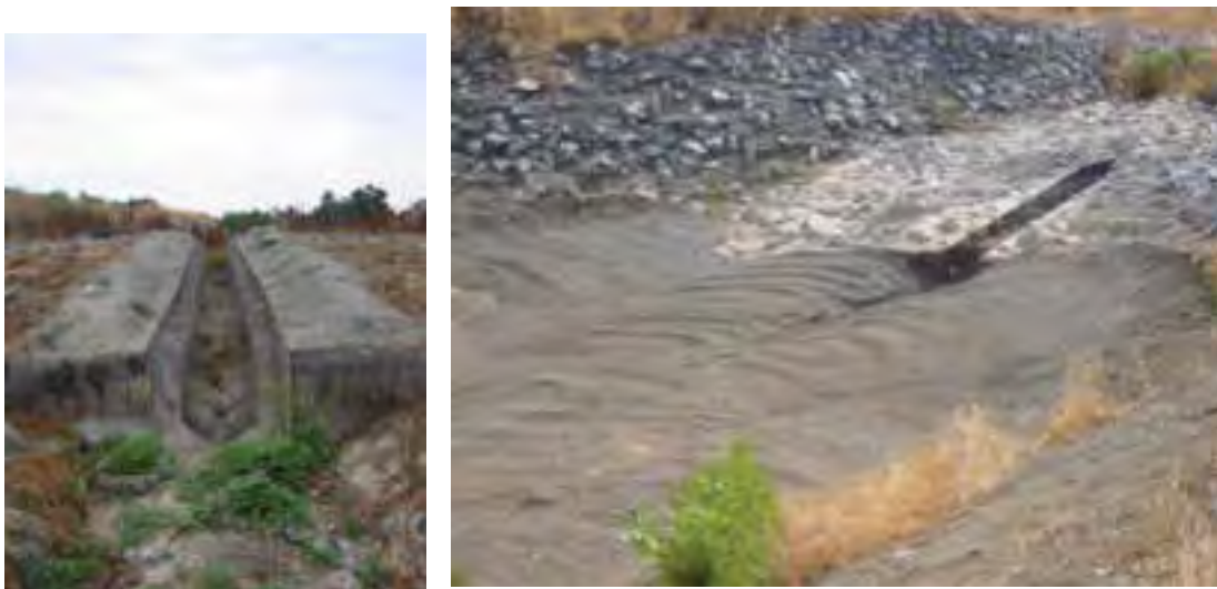
Figure 4.51. Examples of the nine fish ladders, with the sculpted low flow channel, in Llagas Creek north of Pacheco Pass Road.
