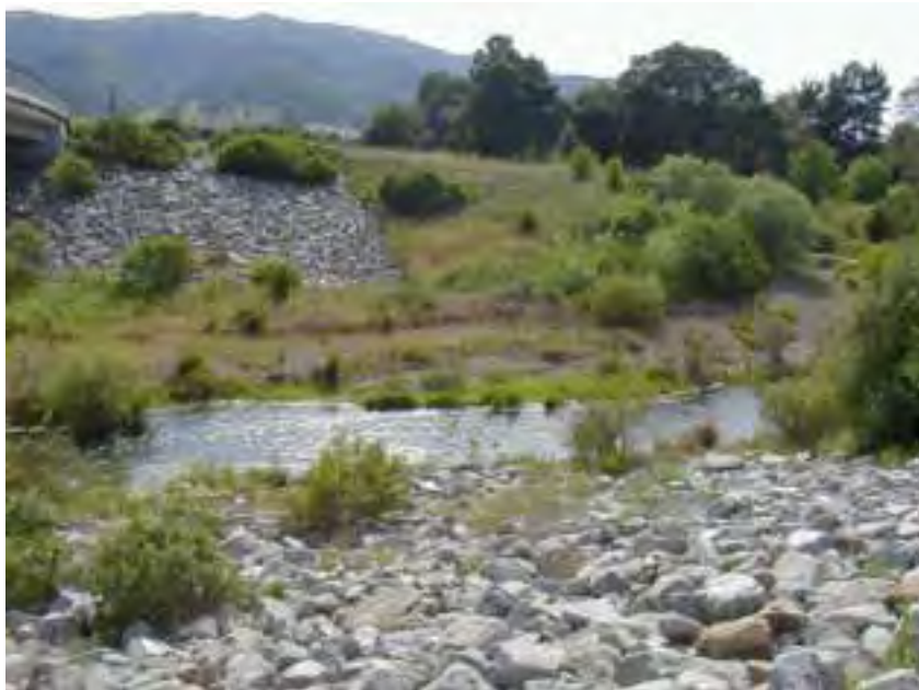
Figure 4.53. Riprap and low flow channel observed on Uvas Creek upstream of West Luchessa Avenue.
