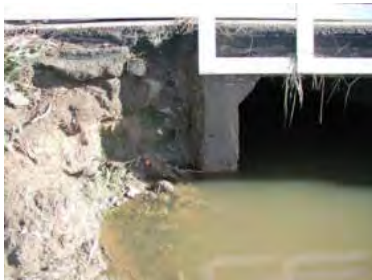
Figure 4.11. Bank erosion and scour pool development south of Watsonville Road on West Little Llagas Creek.
