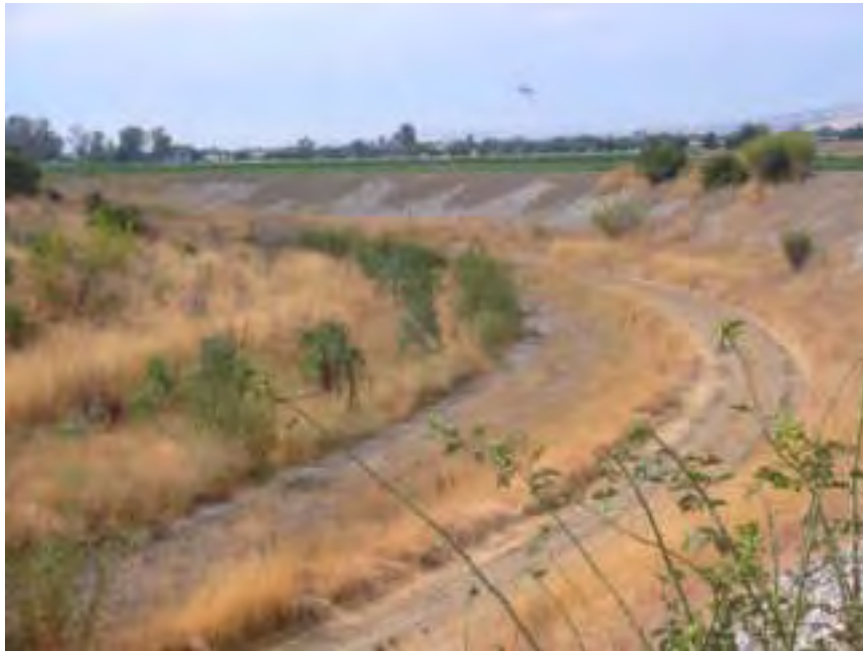
Figure 4.52. Example of engineered Llagas Creek channel with low flow channel, access road, and riprap on channel banks.
