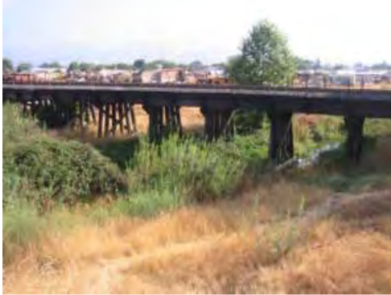
Figure 4.19. Llagas Creek east of Santa Theresa Boulevard at the Southern Pacific Railroad trestle.
