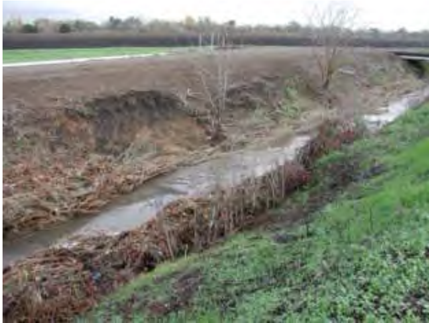
Figure 4.49. Bank slumping on Lower Miller Slough channel.
