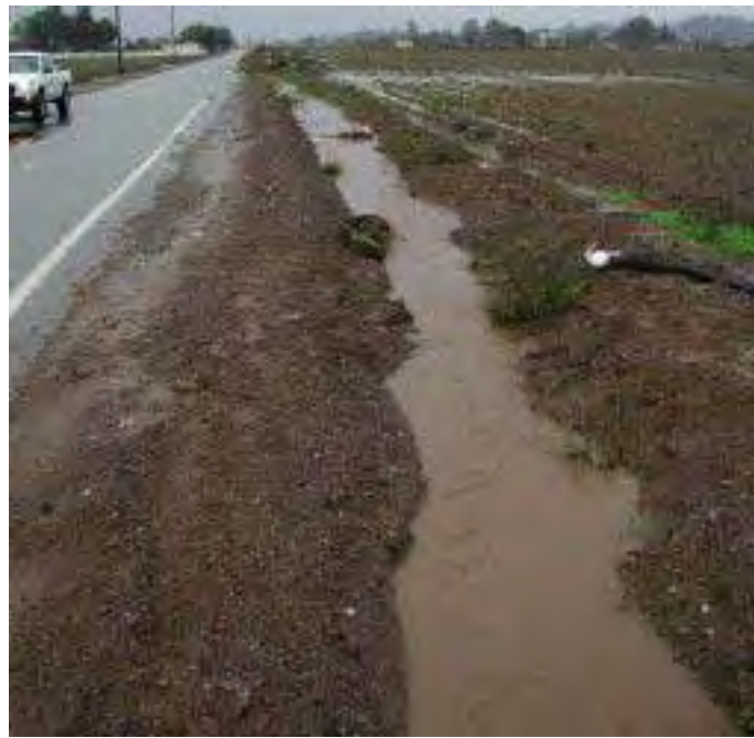
Figure 5.8. Example of Encroachment to Roadway Easements related to Agricultural Drainage Practices.
