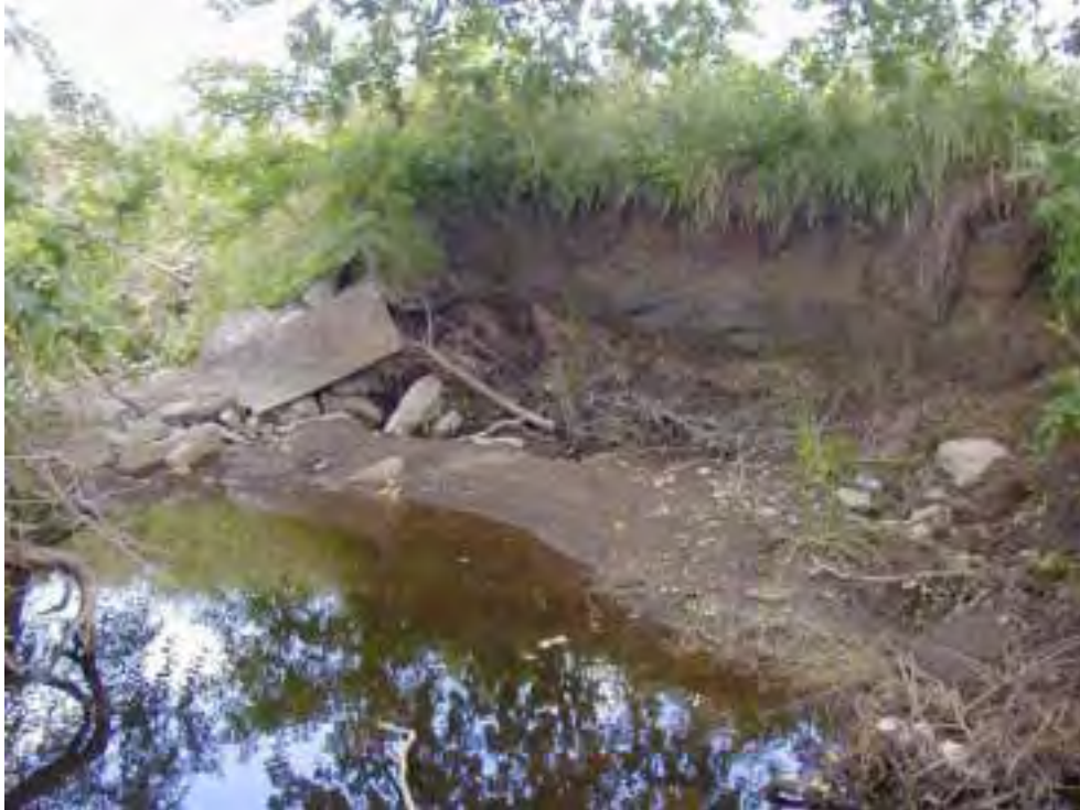
Figure 4.30. Bank scour on West Branch Llagas Creek downstream of Highland Avenue.
