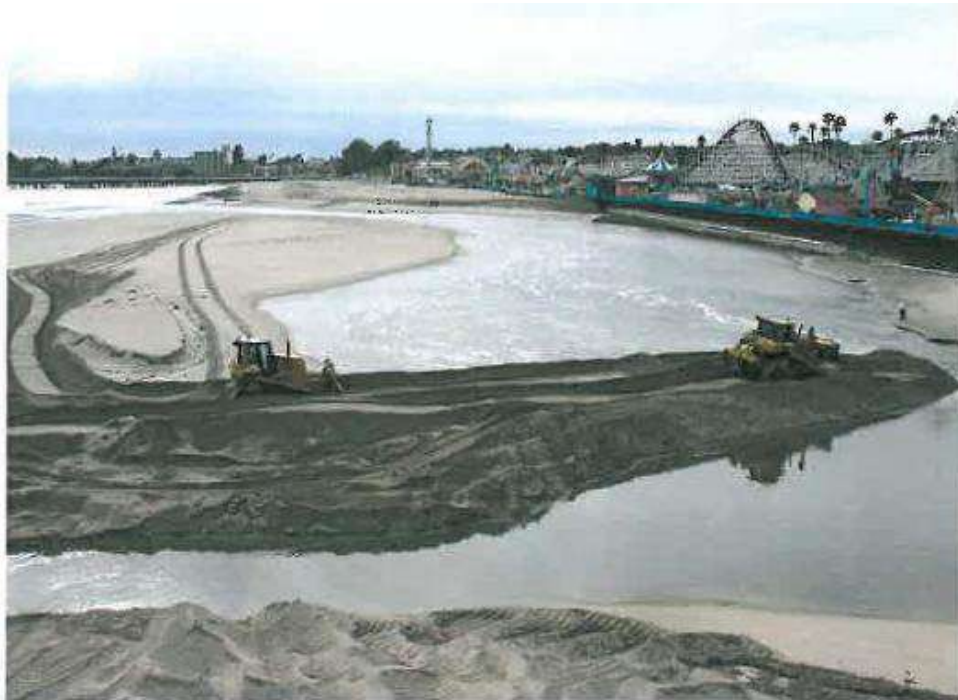
Figure 2-10. Emergency response to redirect the flow of the San Lorenzo River away from Santa Cruz Beach Boardwalk infrastructure (Source: Griggs, 2012)
