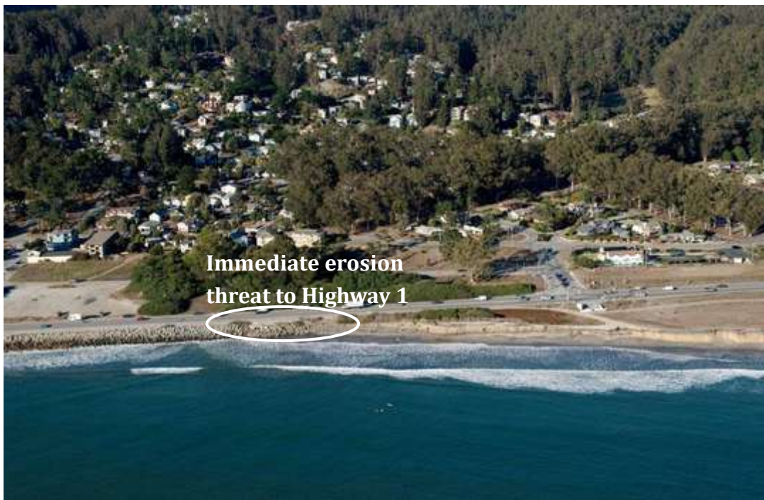
Figure 3-4. Aerial photograph of the northern section of the El Granada County Beach BECA, dated September 2013. Bluff erosion is currently threatening to undermine Highway 1. Source: Adelman and Adelman
